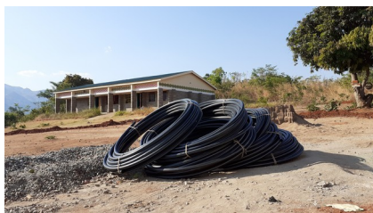
Piping for the water system
